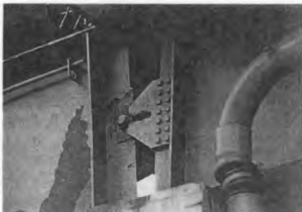
Photo 3 Destruction of the connecting plate
