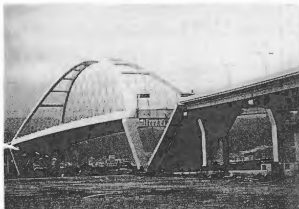
Photo 5 Unseating, side span of the Nishinomiya bridge
